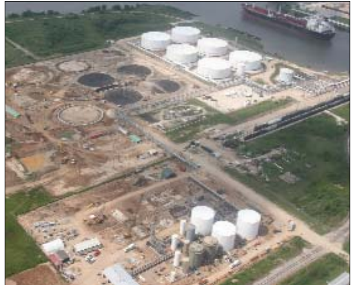
The Green Earth Fuels biodiesel facility is shown under construction in May at the Galena Park terminal in Houston. The construction site can be seen at the bottom of this picture, adjacent to the railroad tracks. Shown at the top of the picture are the feedstock oil and biodiesel storage tanks being built by Kinder Morgan.
